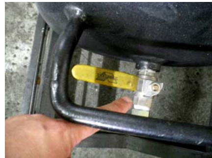
Drainage valve to be opened
