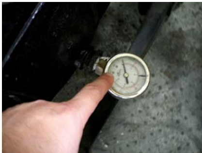
Gauge at 0 pressure level
